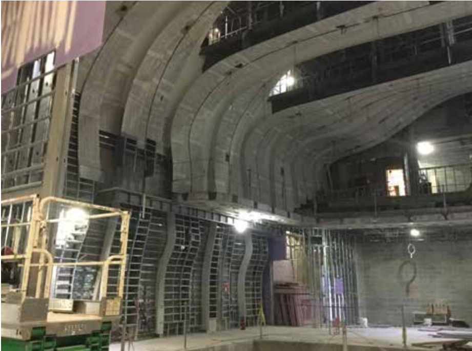
THE TEMPLATE INSTALLATION BELOW THE BALCONIES SERVED AS A GUIDE FOR THE SLOPING AND TWISTING SHAPE CREATED THROUGHOUT THE THEATER.
