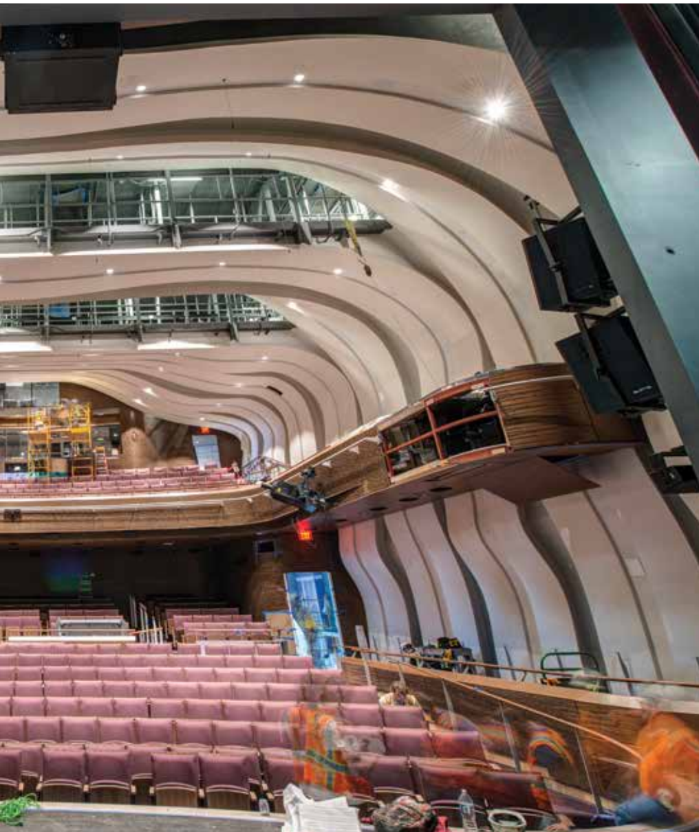
VIEW FROM THE MAIN STAGE OF THE PERFORMANCE HALL, WHERE THE FABRIC HAS BEEN INSTALLED ON THE “RIBBONS,” AND THE THEATER SEATING HAS BEEN FITTED.
